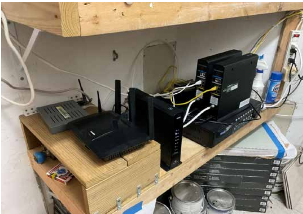
Clubhouse Security Equipment and Wi-Fi
