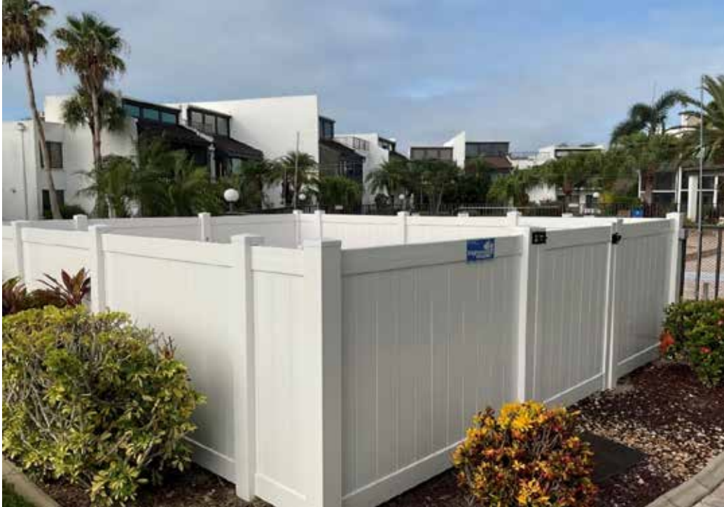
Pool Equipment Fence
