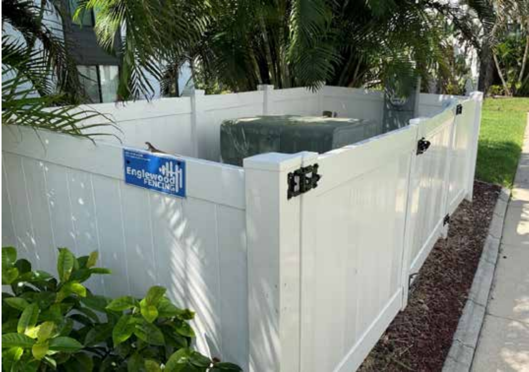
Fence - Gulfside Transformers
