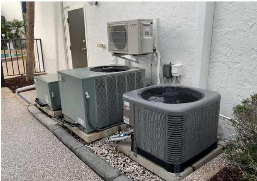
Clubhouse A/C Condensing Units
