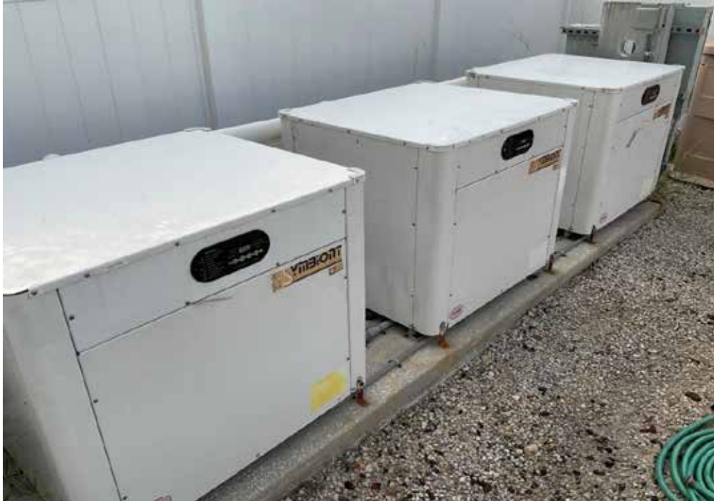
Pool Equipment, Geo-Thermal Heat Pumps
